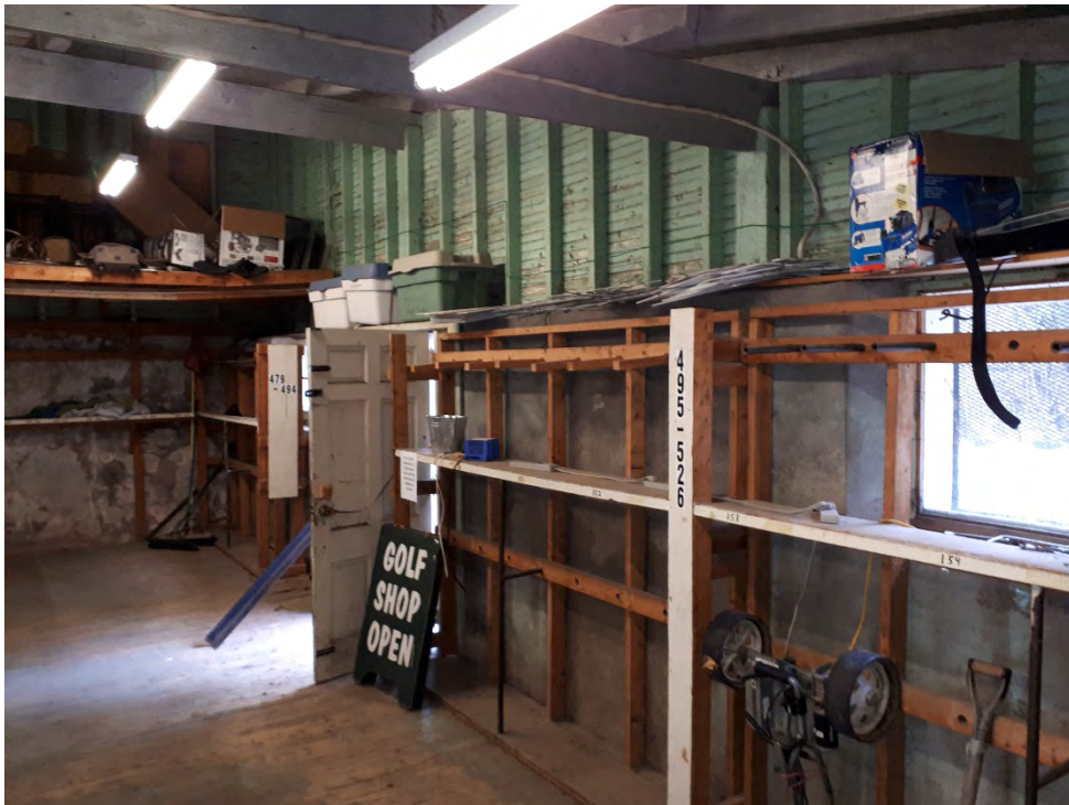
Photo 12 – Green paint in Pro Shop building identified as containing high amounts of lead.
