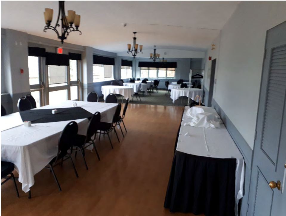
Photo 5 – Banquet hall in club house. Ceiling finishing material identified as asbestos containing.
