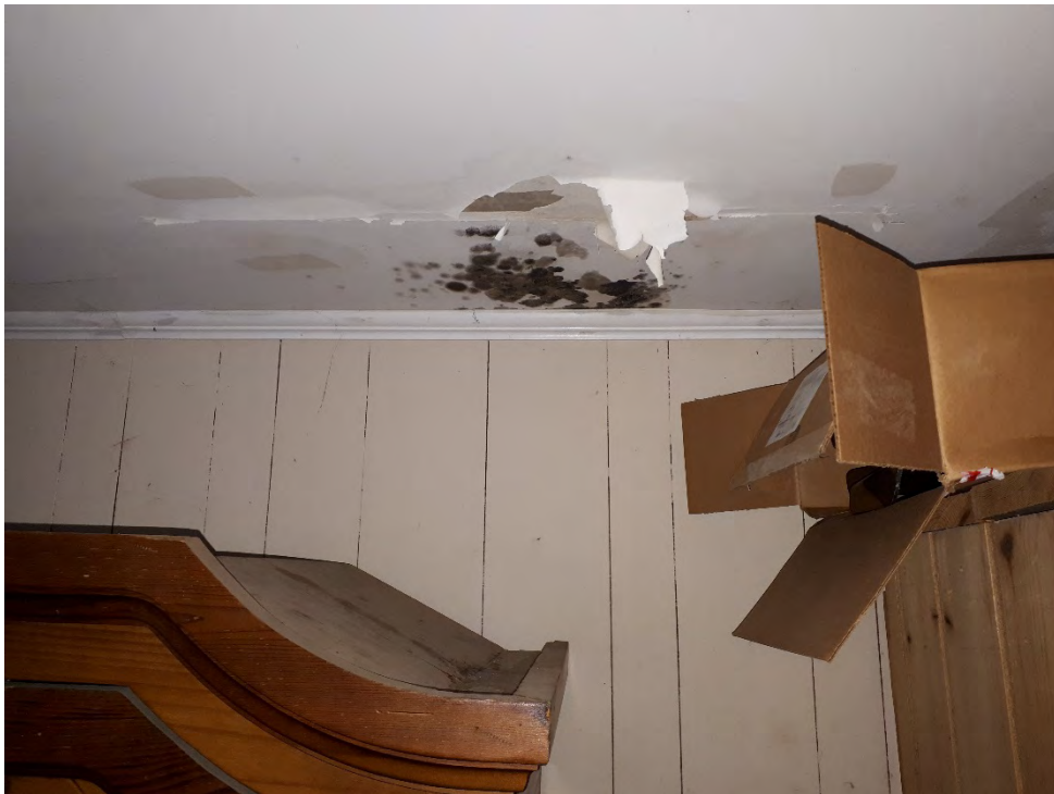
Photo 11 – Mould observed in storage room of Pro Shop. Air sampled in this area (AS-05).
