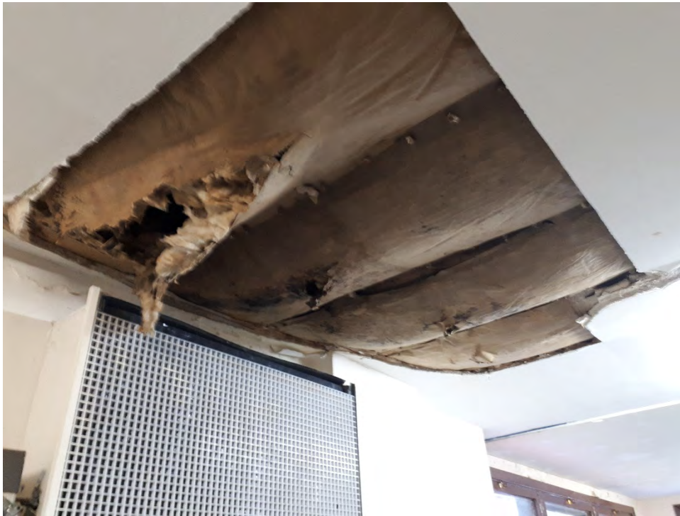
Photo 3 – View of water leak in men's change room.
