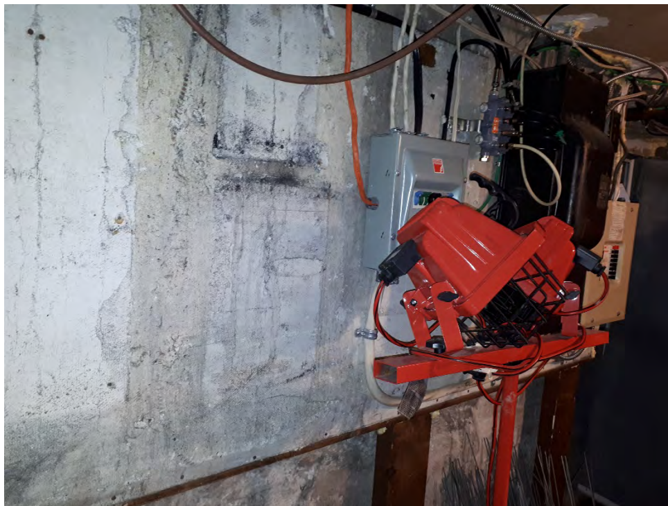
Photo 8 – Paper material on electrical panel in basement of the club house identified as asbestos containing.
