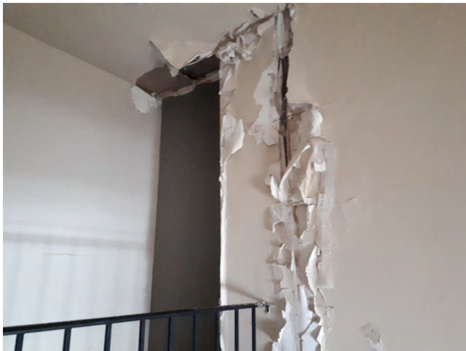
Photo 6 – Peeling of paints observed. Several paints tested were identified as lead based.
